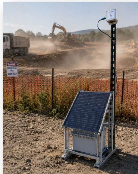
AQ2 Remote Monitoring Station
